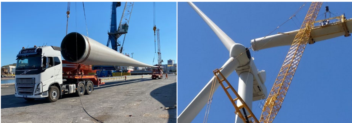
In Piombino, an entire set of rotor blades had to be replaced after sustaining lightning damage.
