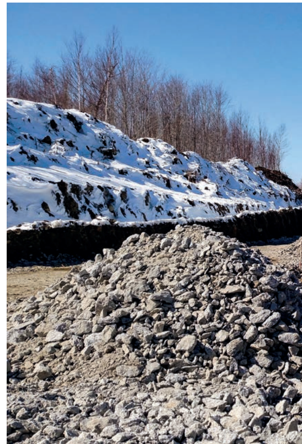
Preparation work for the wind farm Pisgah Mountain: new road construction is making the future sites accessible
